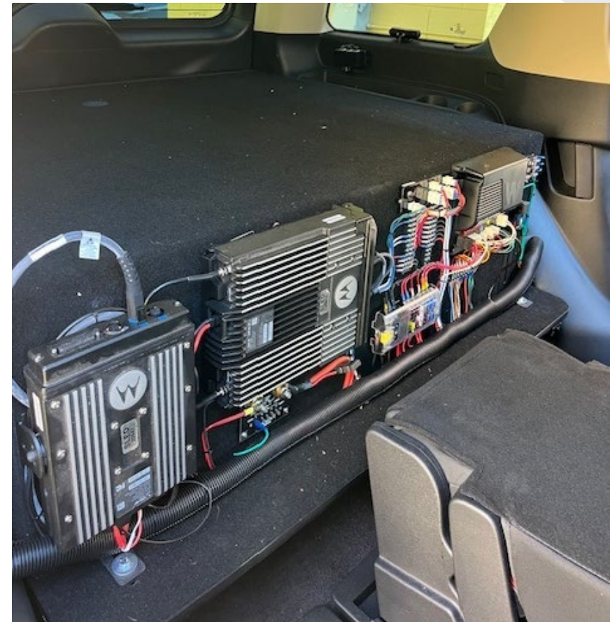
Regional Investigator-SUV radio, siren, & emergency lighting controllers.
